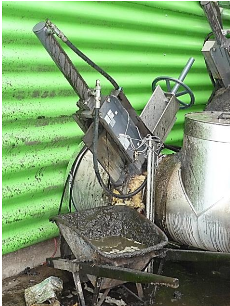
Outlet / inlet side of the digester....yesterday
