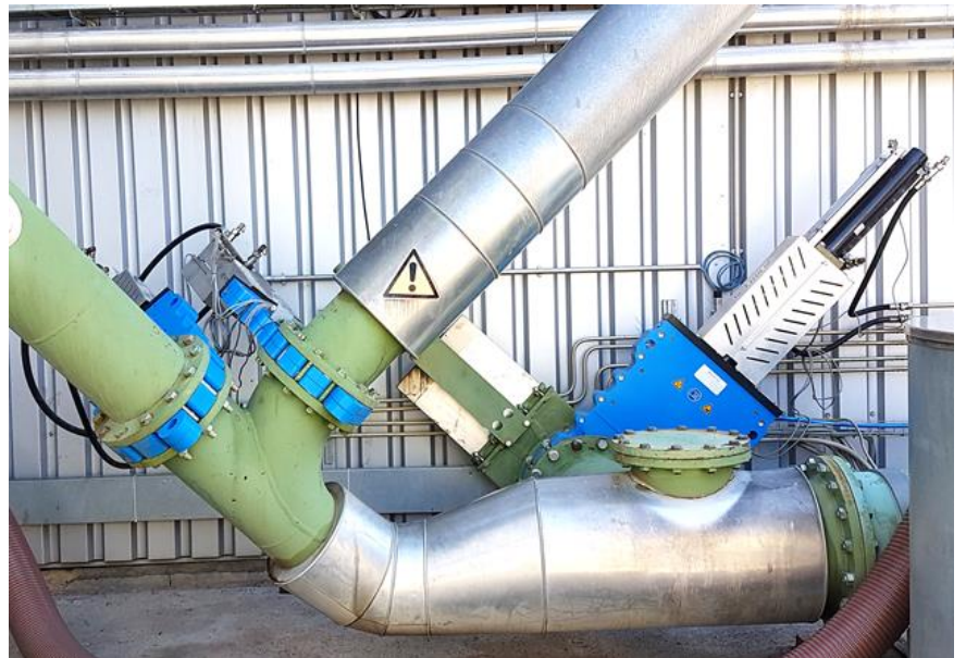
Digester outlet / inlet.....today
